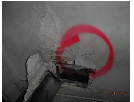
Sample 2-1 Duct Wrap
