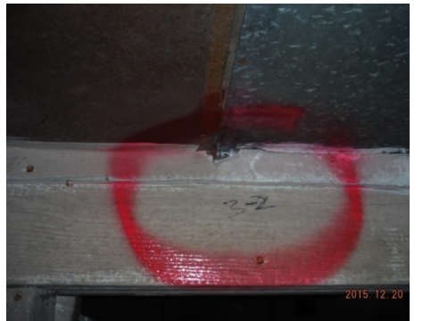
Sample 3-2 Duct Wrap
