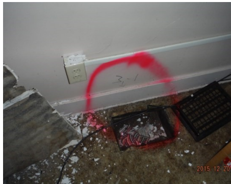
Sample 3-1 Duct Wrap
