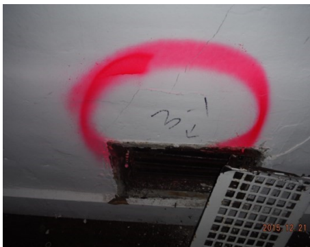
Sample 3-1 Duct Wrap
