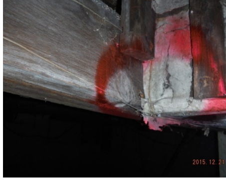
Sample 3-2 Duct Wrap
