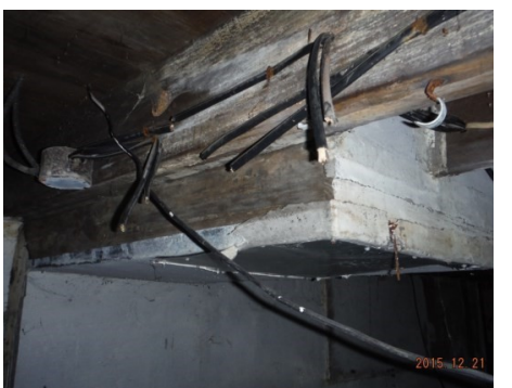
Additional Duct Wrap Located in Basement
