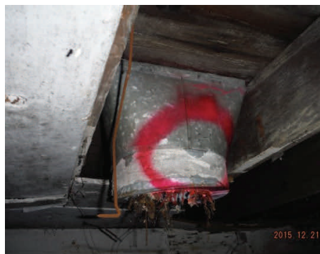
Sample 6-1 Duct Wrap
