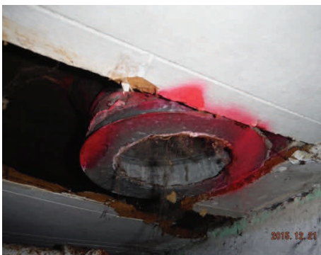
Additional Duct Wrap in Basement
