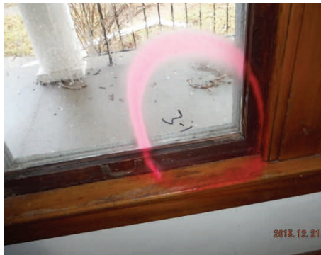
Sample 3-1 Window Glazing
