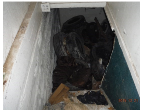
Clutter around basement steps
