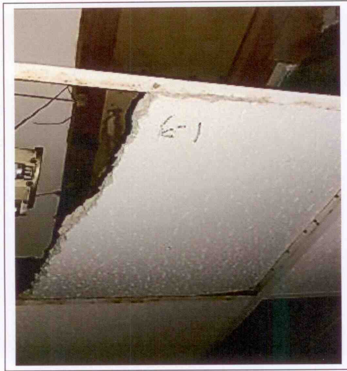
2'x4' Suspended ceiling tile ceiling tile with holes and fissures
