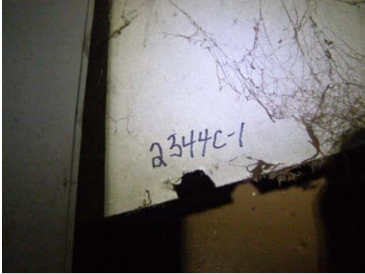
Photo 1: Furnace Board (2344C-1) Kitchen, Ceiling. 45% Chrysotile Asbestos Detected.
