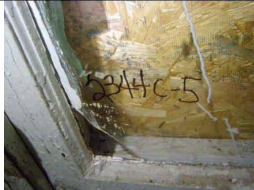
Photo 4: Window Glazing (2344C-5) Living Room, Wall D. 2% Chrysotile Asbestos Detected (PC=1.25%).
