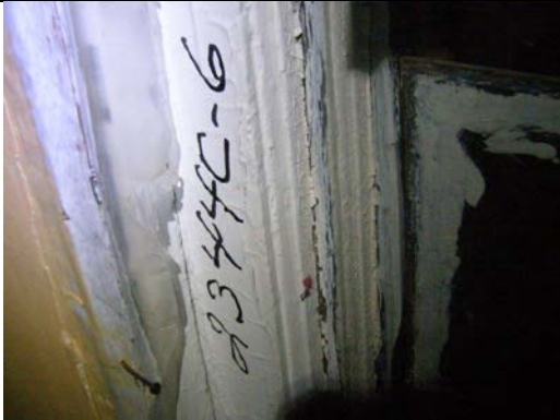
Photo 5: Window Glazing (2344C-6) Bedroom 1, Wall B. 2% Chrysotile Asbestos Detected (PC=1.25%).
