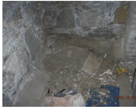
Transite on Floor in Basement
