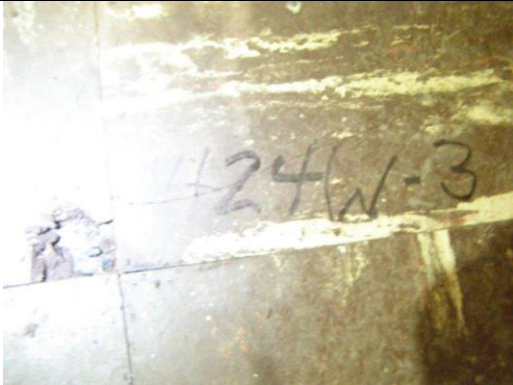
Photo 3: Floor Tile (1424W-3) Living Room, Floor. 5% Chrysotile Asbestos Detected (PC=3.25%).
