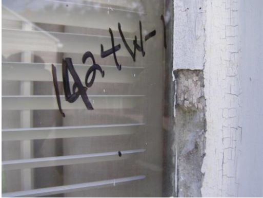
Photo 1: Window Glazing (1424W-1) Exterior, Wall B. 2% Chrysotile Asbestos Detected (PC=1.50%).
