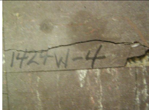
Photo 4: Floor Tile (1424W-4) Bath Hall, Floor. 5% Chrysotile Asbestos Detected (PC=4.25%).
