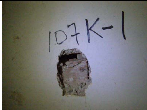
Photo 10: Plaster (107K-1) Dining Room, Wall B. Trace <1% Chrysotile Asbestos Detected (PC=0.50%).
