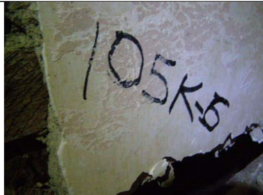
Photo 6: Plaster (105K-6) Dining Room, Wall D. Trace <1% Chrysotile Asbestos Detected (PC=<0.25%).
