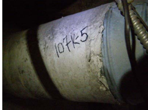
Photo 14: Duct Work Wrap (107K-5) Basement, Ceiling. 65% Chrysotile Asbestos Detected.
