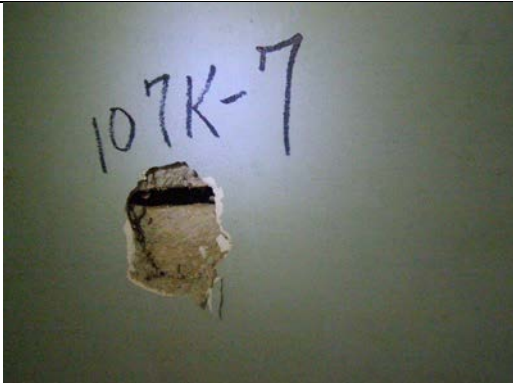
Photo 15: Plaster (107K-7) Bedroom 2, Wall B. Trace <1% Chrysotile Asbestos Detected PC=<0.25%).
