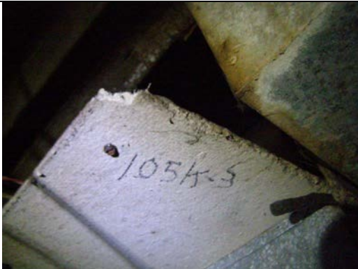
Photo 3: Furnace Board (105K-3) Basement. 68% Chrysotile Asbestos Detected.
