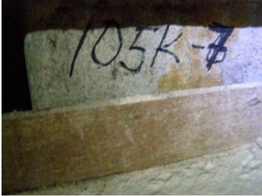
Photo 7: Duct Work Wrap (105K-7) Dining Room 65% Chrysotile Asbestos Detected.
