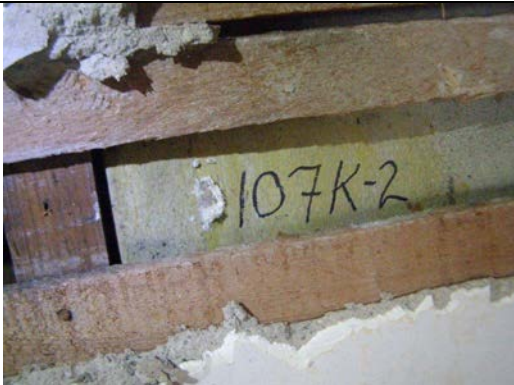
Photo 11: Duct Work Wrap (107K-2) Dining Room, Wall B. 65% Chrysotile Asbestos Detected.
