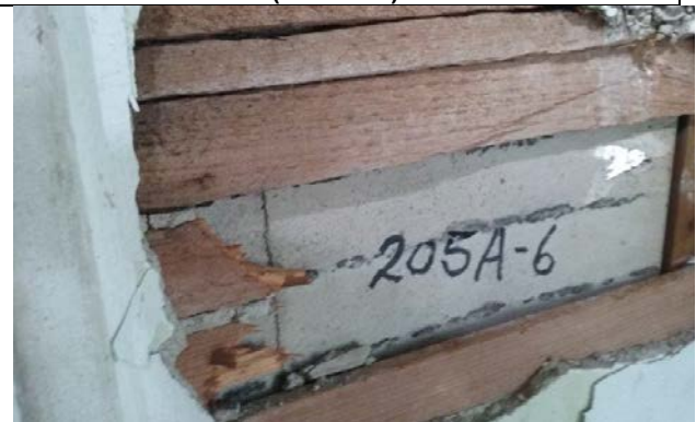
Photo 6: Duct Work Wrap (205A-6) Dining Room, Wall D. 70% Chrysotile Asbestos Detected.
