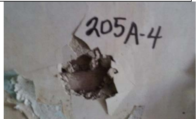
Photo 4: Plaster (205A-4) Kitchen, Wall D. Trace <1% Chrysotile Asbestos Detected (Base Coat) (PC=0.25%).
