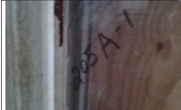
Photo 1: Window Glazing (205A-1) Living Room, Wall A. Trace <1% Chrysotile Asbestos Detected (PC=0.50%).
