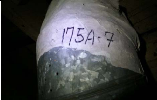
Photo 7: Boot Wrap (175A-7) Basement. 65% Chrysotile Asbestos Detected.
