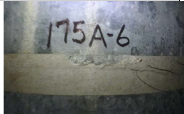
Photo 6: Seam Tape (175A-6) Basement, Ceiling. 80% Chrysotile Asbestos Detected.
