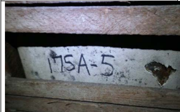
Photo 5: Duct Work Wrap (175A-5) Family Room, Wall B. 65% Chrysotile Asbestos Detected.
