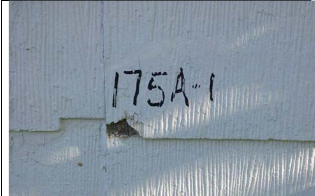
Photo 1: Transite (175A-1) Exterior. 20% Chrysotile Asbestos Detected.
