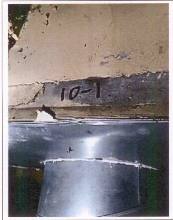
HA #10 – Duct insulation
