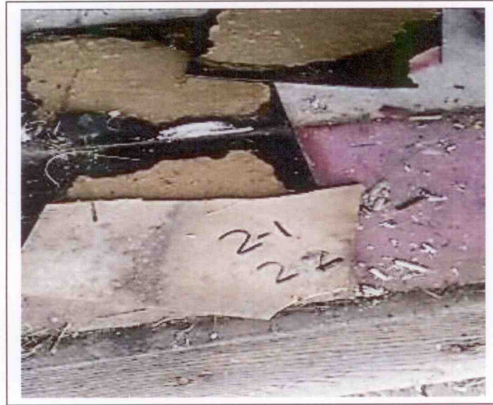
HA #2, #3 – 9”x9” Tan floor tile with black mastic
