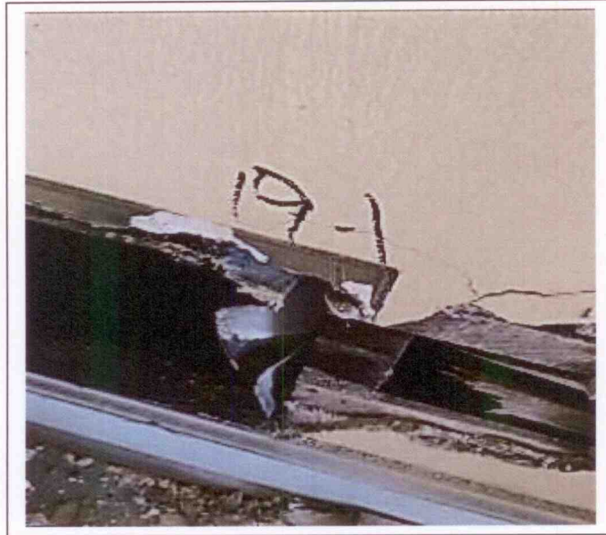
HA #19 – Duct insulation concealed behind hard wall plaster
