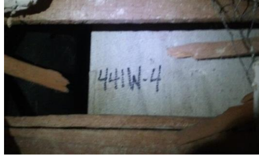
Photo 4: Duct Work with Wrap (441W-4) Kitchen, Wall A. 65% Chrysotile Asbestos Detected.
