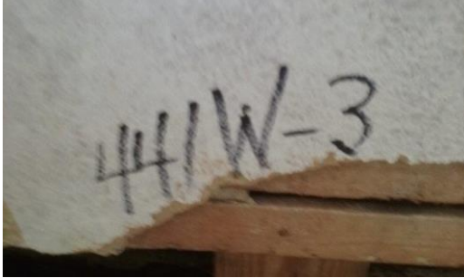
Photo 3: Plaster (441W-3) Living Room Closet, Wall C. Trace <1% Chrysotile Asbestos Detected (PC=0.25%).
