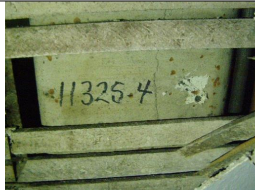
Photo 4: Duct Work Wrap (1132S-4) Living Room, Wall B. 65% Chrysotile Asbestos Detected.
