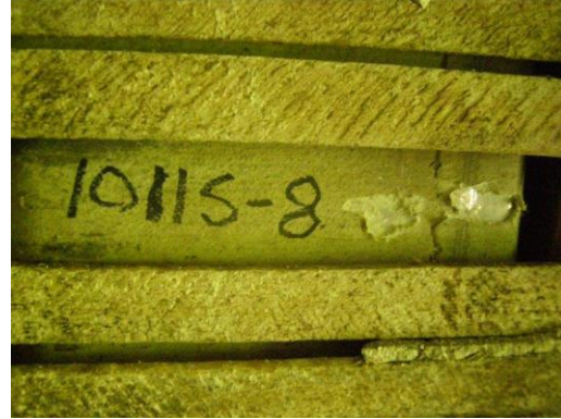
Photo 8: Duct Work Wrap (1011S-8) Entry. 65% Chrysotile Asbestos Detected.
