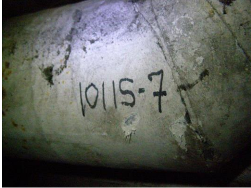
Photo 7: Duct Work Wrap (1011S-7) Basement. 45% Chrysotile Asbestos Detected.
