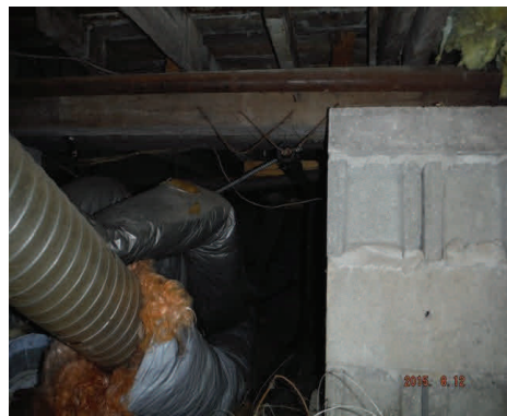
Duct work in Basement
