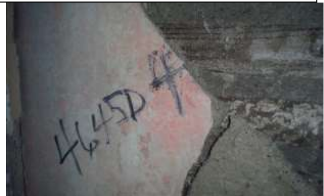
Photo 4: Plaster (4645D-4) Dining Room, Wall D. Trace <1% Chrysotile Asbestos Detected (PC=<0.25%).
