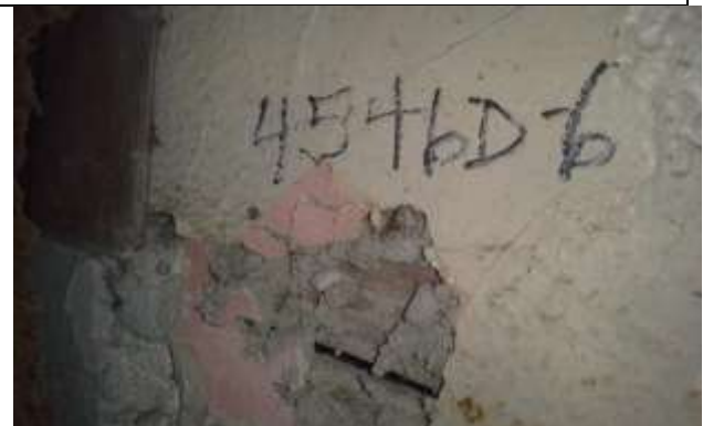
Photo 6: Plaster (4645D-6) Bedroom 2, Wall D. Trace <1% Chrysotile Asbestos Detected (PC=0.25%).
