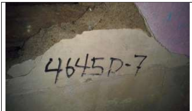
Photo 7: Plaster (4645D-7) Bedroom 1, Wall D. Trace <1% Chrysotile Asbestos Detected (PC=<0.25%).
