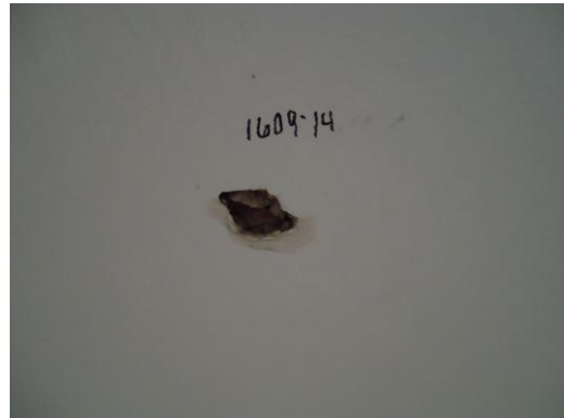
Photo 14: Ceiling Plaster. (1609-14) Bath. No Asbestos Detected.
