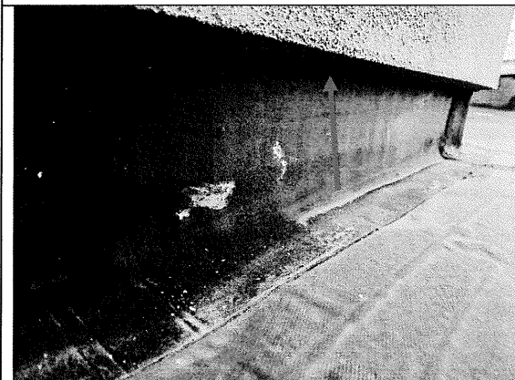
33 – EPDM base flashing at roof monitor wall – note no termination of the EPDM, simply extends behind EIFS.
