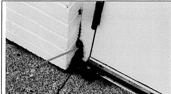
17 – Rusting of the hollow metal door frame at the man door at the east warehouse
