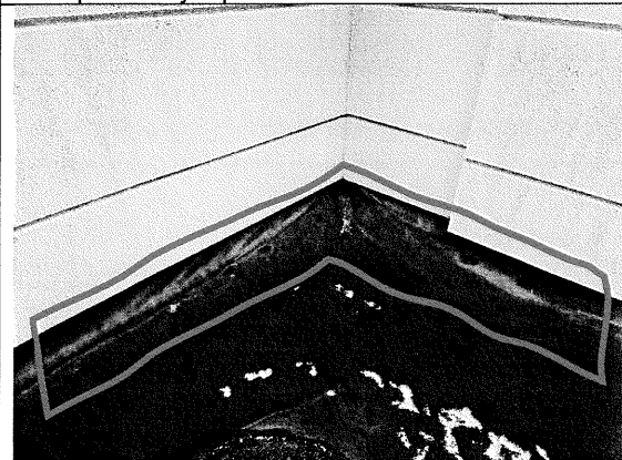
47 – Note pulling of the base flashing at the original building roof at the roof monitor.
