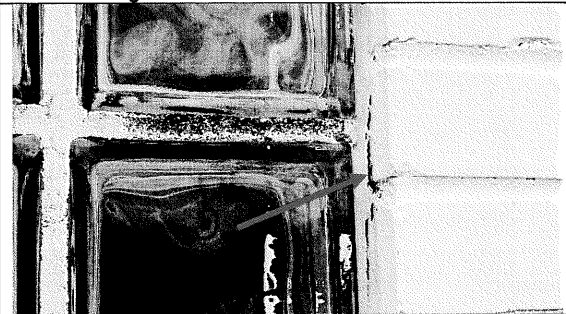
16 – Sealant failure at the perimeter of the glass block opening at the east warehouse
