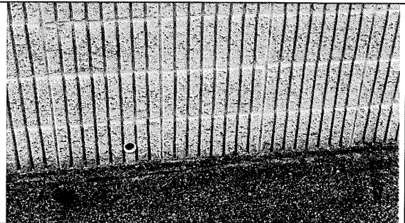
06 – Typical ribbed CMU at planters at base of original portion of the building
