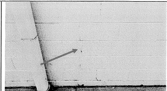
18 – existing CMU facades with vertical and stair step cracking in select areas
