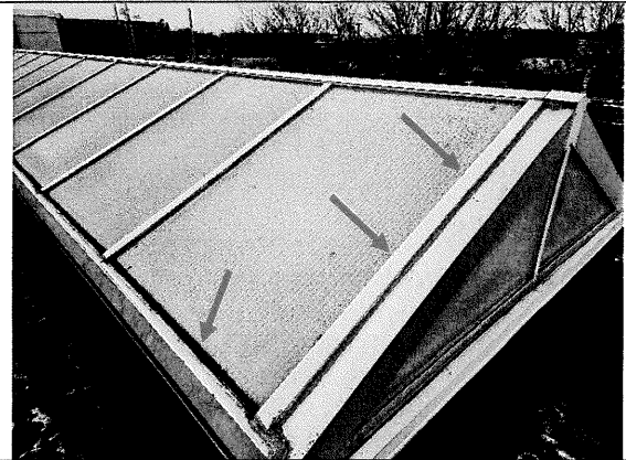
44 – Typical skylight conditions – glazing is nearing the end of its service life, joint sealant applied to maintain water tight.
