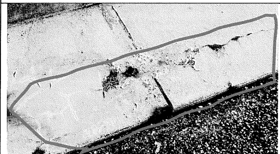
23 – Northwest Entrance – surface rust on the concrete likely from proximity of the reinforcing steel to the surface of the concrete.
