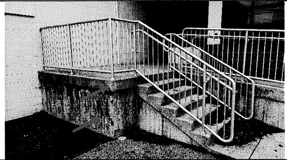
26 – South Entrance – failing concrete parge coat at face of vertical concrete surfaces.
