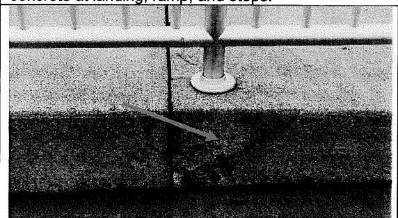
24 – Northwest Entrance – Existing railing system / spalled concrete at railing post bases.
