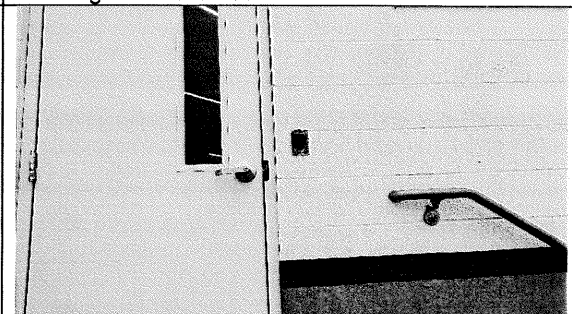
20 – existing CMU facades with vertical and stair step cracking in select areas
