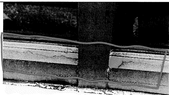
07 – aluminum storefront system – painted finishes are failing exposing the original colored anodized finish
