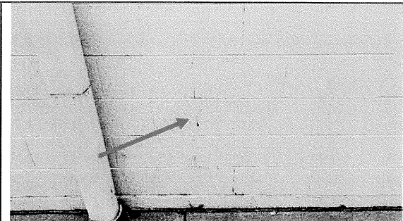
18 – existing CMU facades with vertical and stair step cracking in select areas
