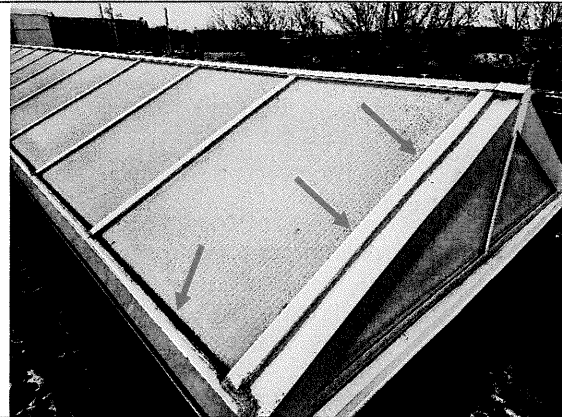
44 – Typical skylight conditions – glazing is nearing the end of its service life, joint sealant applied to maintain water tight.
