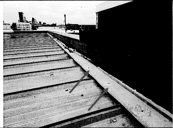
38 – head / high wall flashing at the south warehouse. Note the exposed fasteners at the flashing have been repaired. The flashing is exhibiting some rust.
