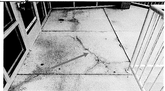
22 – Northwest Entrance – cracking and spalled concrete at landing, ramp, and steps.
