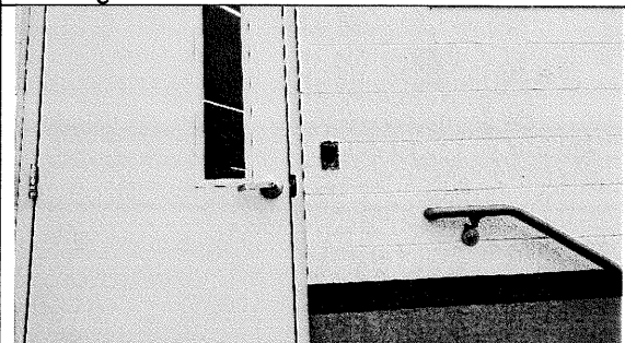
20 – existing CMU facades with vertical and stair step cracking in select areas
