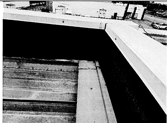
46 – EPDM wase flashing over CMU parapet walls, capped with metal coping at south warehouse roof.
