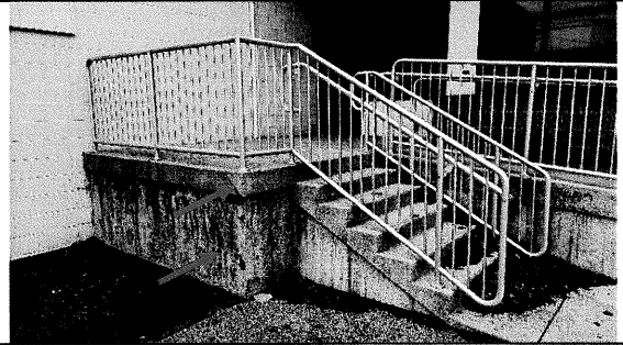
26 – South Entrance – failing concrete parge coat at face of vertical concrete surfaces.
