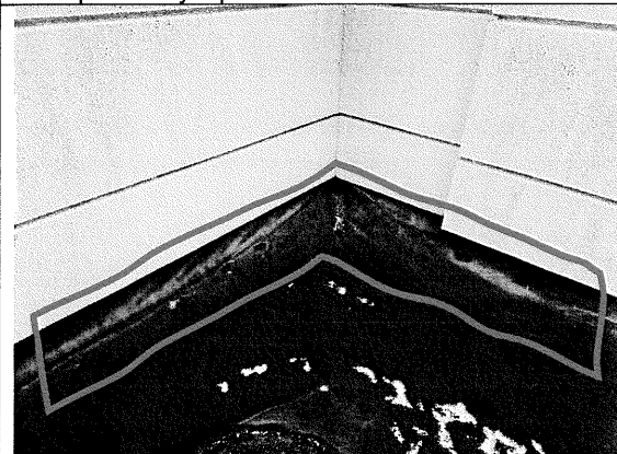
47 – Note pulling of the base flashing at the original building roof at the roof monitor.
