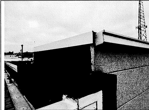
37 – Transition between upper roof monitor and the base flashing at the north side of the south warehouse
